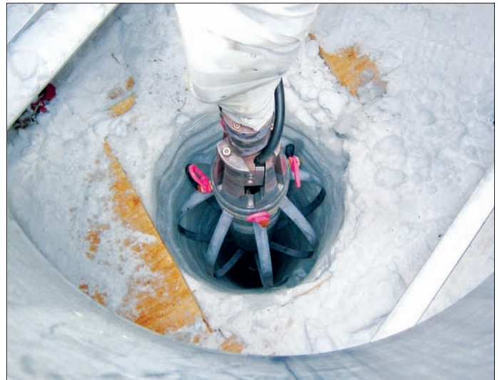
The drill head being removed from Hole 80, the final IceCube hole to be drilled. (Image credit: Jim Haugen.)
